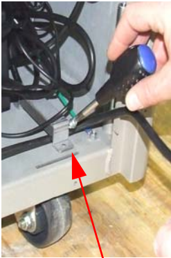
UPS power cable secured by bracket
