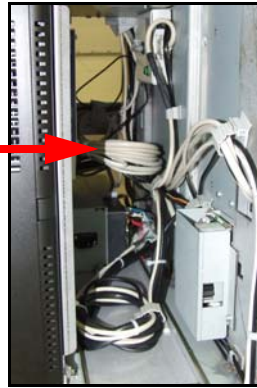
Service loop, as seen from the front of the Station
