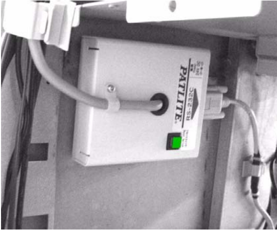
Orientation: Logic Box seen from back of Station.
