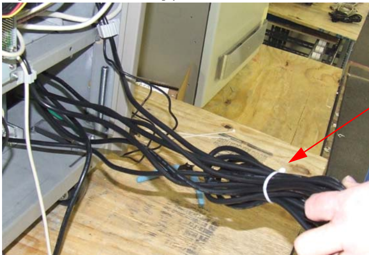
service loop, secured with tie wrap (rear view)
