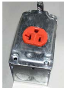
isolated ground junction box
