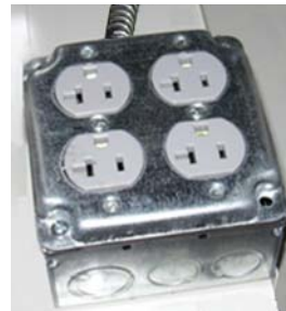
unregulated power junction box
