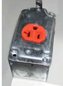
isolated ground junction box
