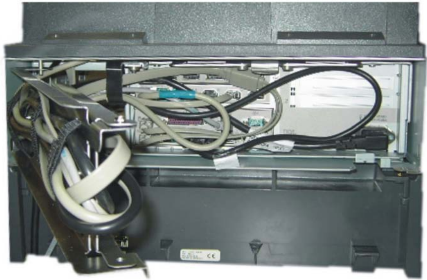
Figure 82. Cable assembly arm with cables securely in place
